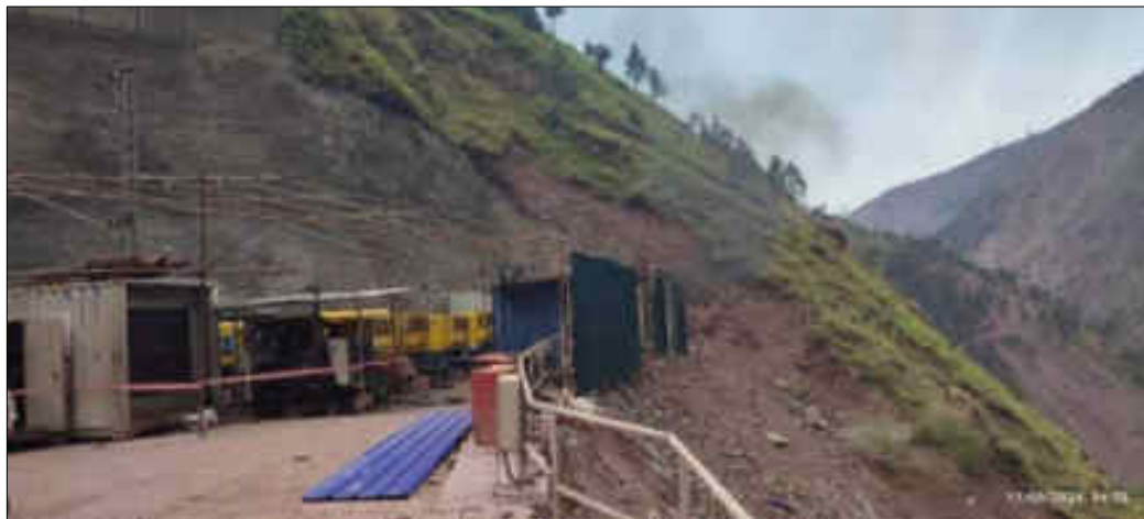
Emission from diesel generator at the Adit tunnel A3.
