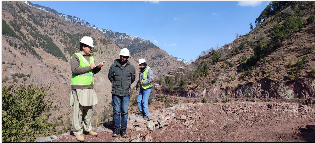
Recording non-compliances at Adit-3 site (January 26, 2023)
