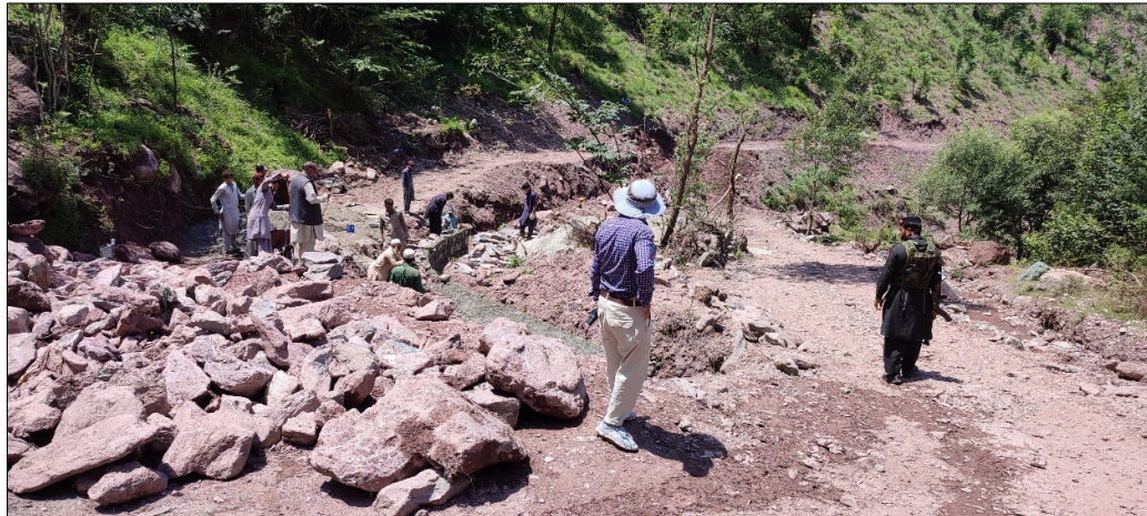
Non-compliance - Work without PPE on temporary access road to Adit 3 (August 04, 2022)
