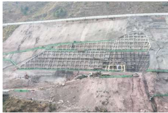
Fixing of the Frame Beam at the Left Abutment of the Dam
